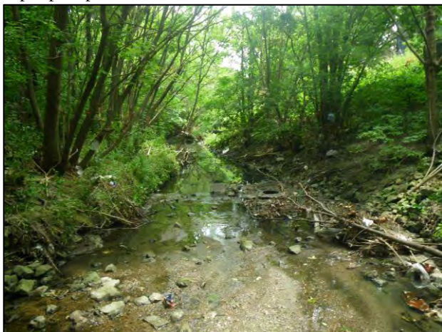
Facing downstream (southeast) at watercourse directly downstream of culverts. Banks in this area lined with gabion baskets (note loose stones from broken baskets)
