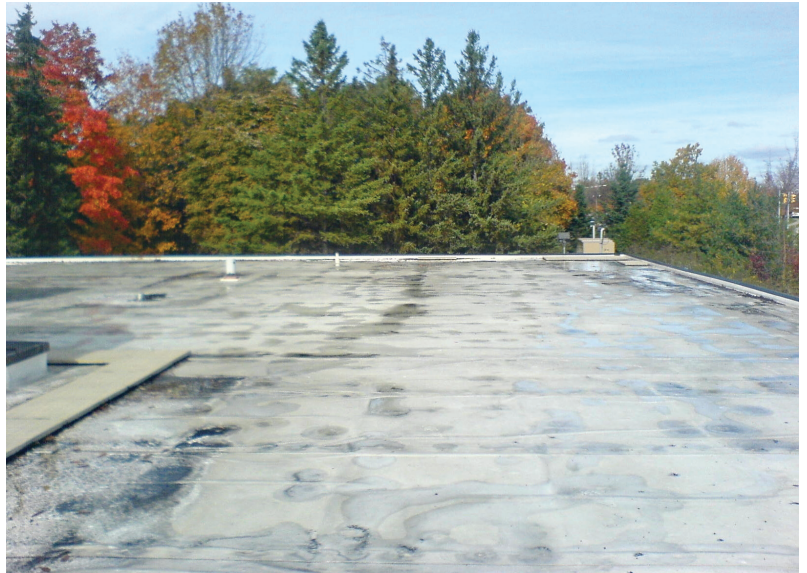
Black Creek Pioneer Village installed its cool roof in 2009
